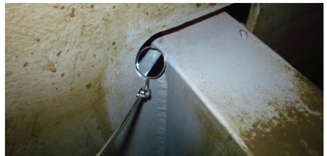
Top image: Water ballast tank after 10 years of service
