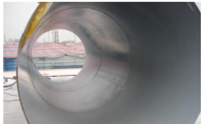
Top image: Initial pipe condition
