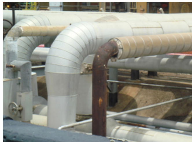
Corrosion Under Insulation (CUI)
