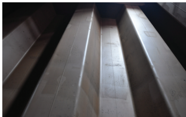
Top image: PHENGUARD-coated tanks in excellent condition after 12 years in service Bottom image: 12 years of maximum resistance in a chemical tanker
