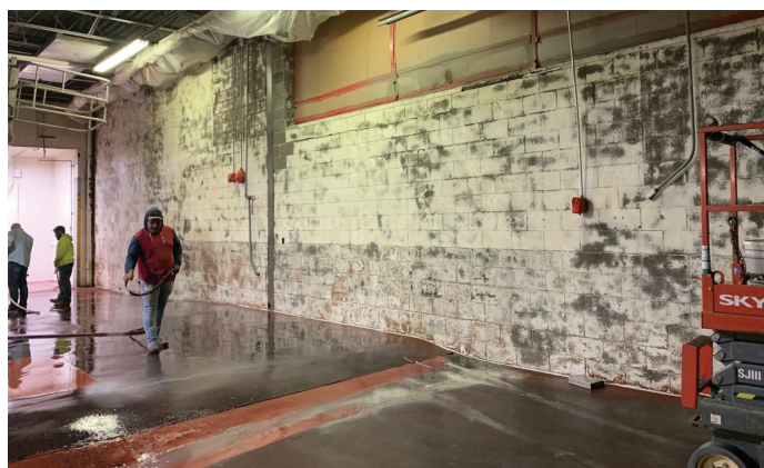
Surface preparation included removal of fiberglass reinforced panels and sandblasting multiple layers of damaged coatings.
